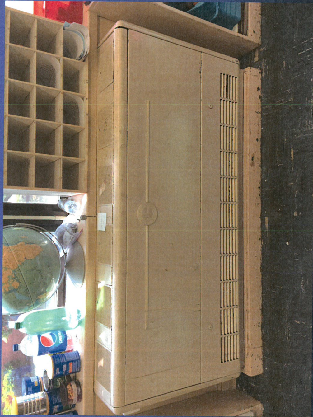
Existing Unit Ventilators
